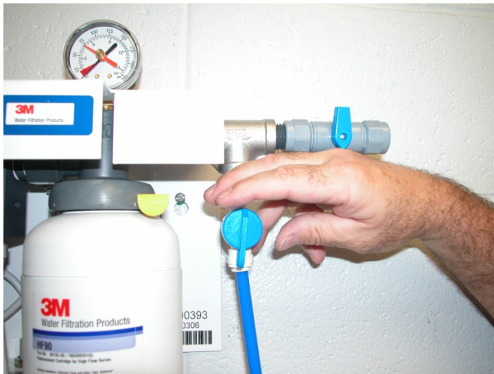
Open/Close outlet sample valve
