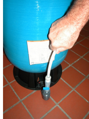
Open tank valve
