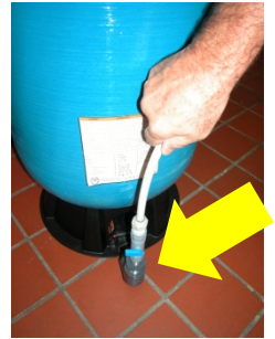
Turn Off tank line
