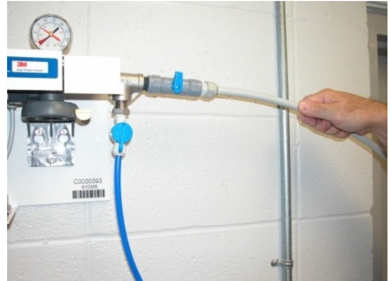
Outlet to equipment water supply
