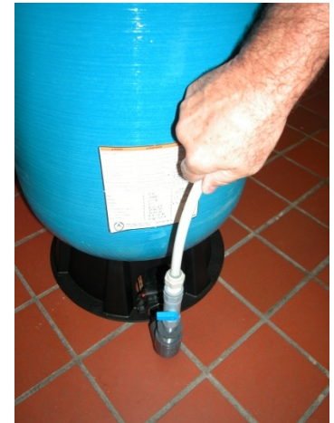
Tank line connection at Tank
