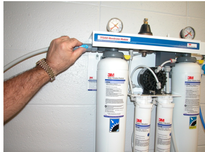
Open inlet water line
