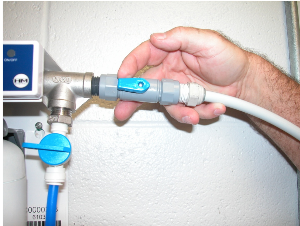
Open outlet water line
