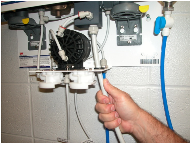
Tank line connection on Unit
