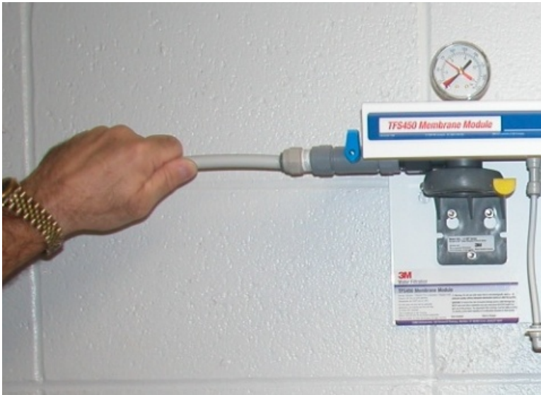
Inlet water supply
