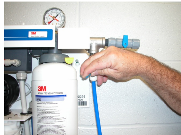
Open outlet sample valve
