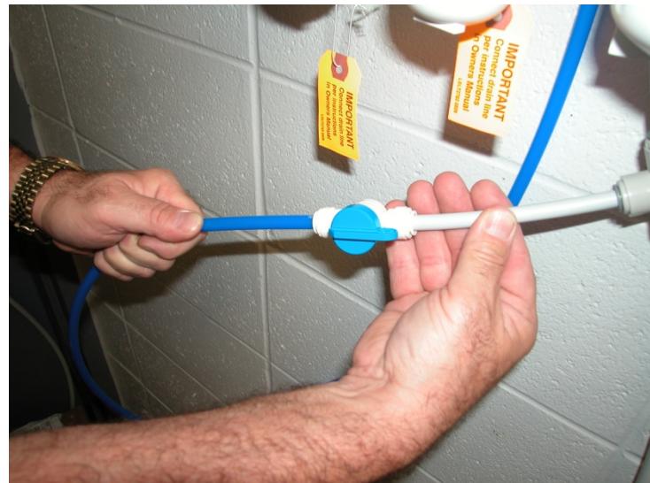
Open/Close tank line sample valve
